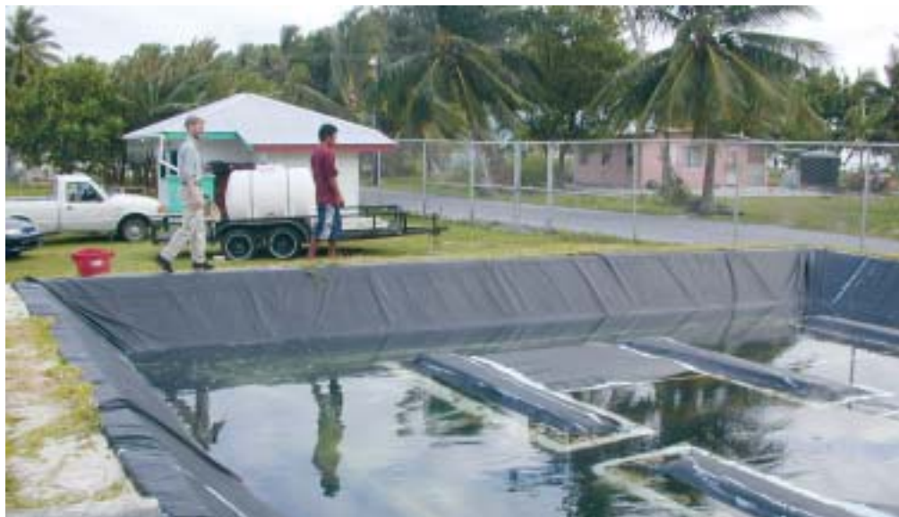
A water treatment plant, part of an ADB project to improve water and sanitation facilities.
